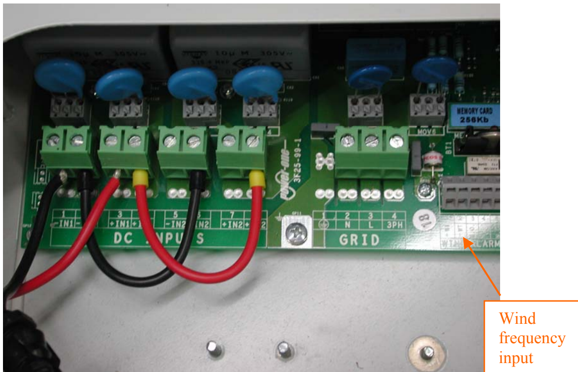
Fig.12 - DC section cables
